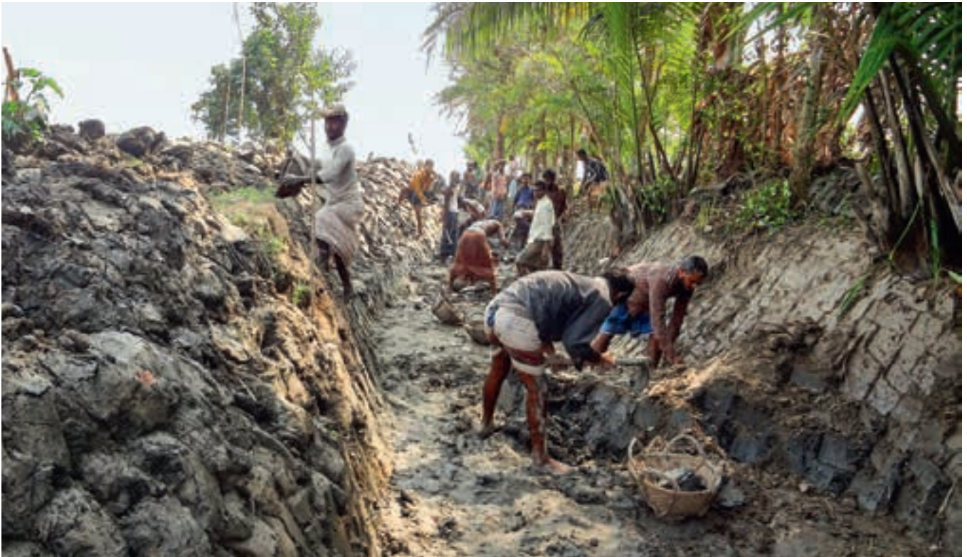
Social mobility is also part of the project: instead of waiting for government help, some villagers dig ditches themselves or repair dikes to protect their land from flooding.
